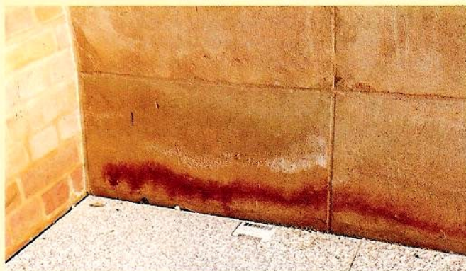
Discoloration and staining spoils the all-important look of stone. Shown here are the spread of the oxidation of pyrite in slate on a roof (top), bedding materials on granite (middle) and staining on limestone.
