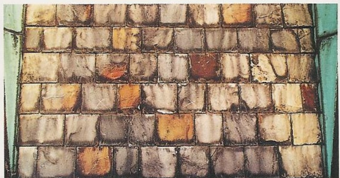
Slate roofing in central London showing discolouration due to reaction with some acidic components of rain. There are also dirt deposits.
